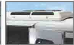
Rooftop Mounted AC
